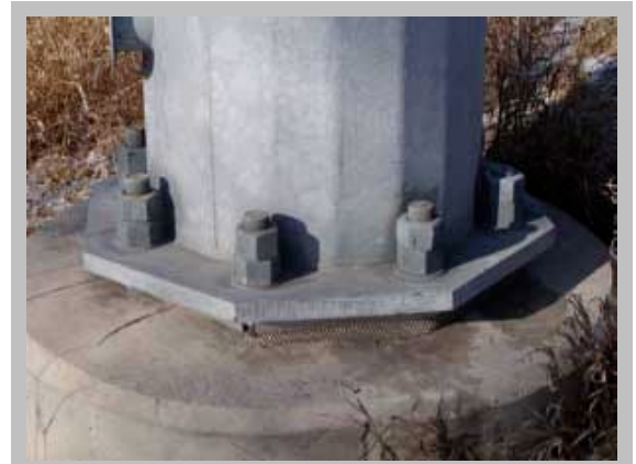
Inspection of base plate anchor rods was found to be critical.
