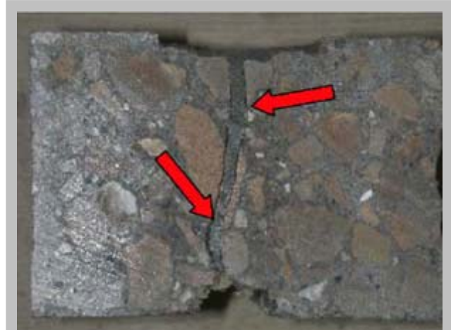
Crack sealant tests included bond strength and durability. One failure mode, cracking between the sealant and the concrete, is indicated by the red arrows.
