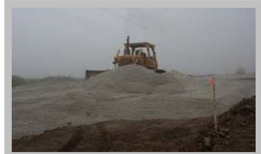
Use of foundry slag is one of many subgrade improvement options in Wisconsin.
